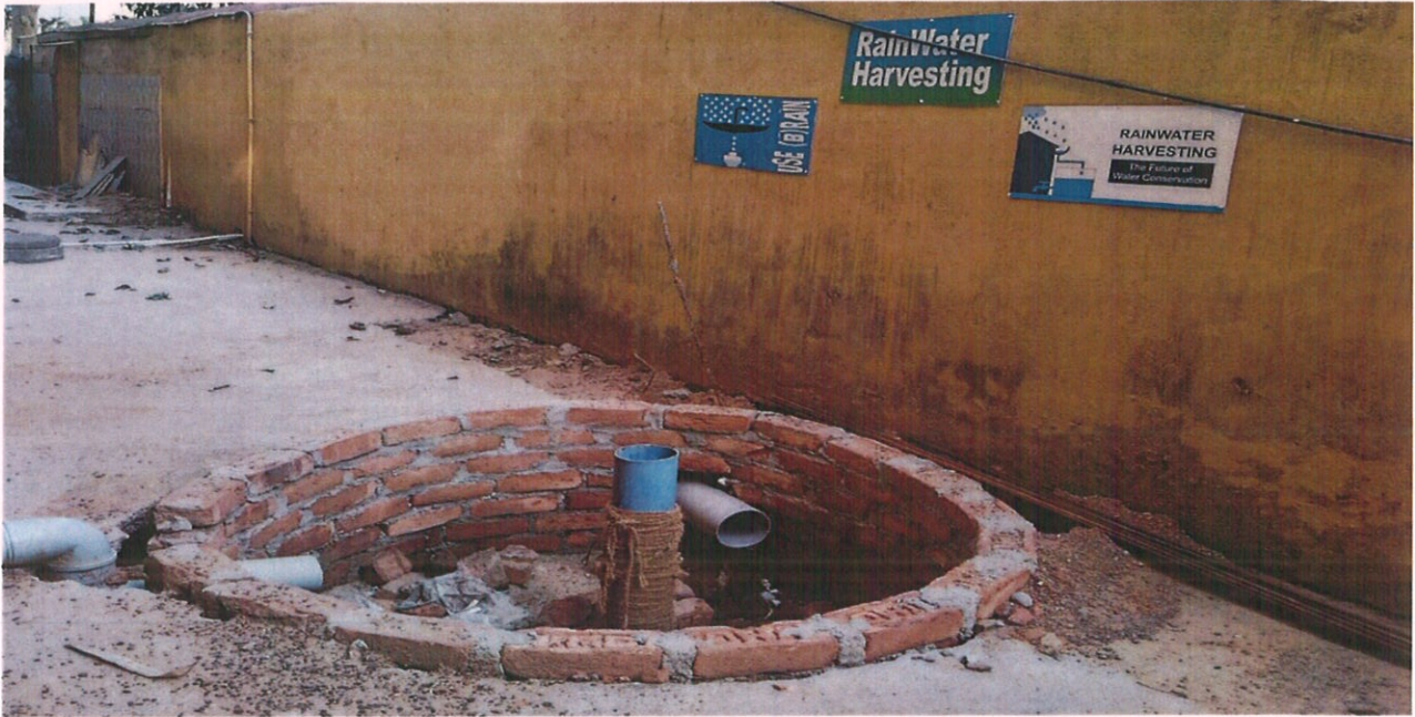
Rain Water Harvesting in the campus of NSU
