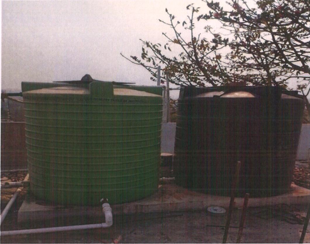
Water tanks in Chandrasekhar block
