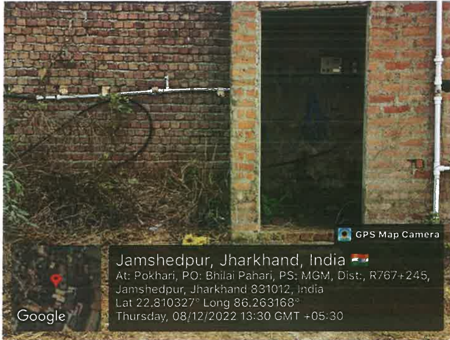
Waste water recycling center
