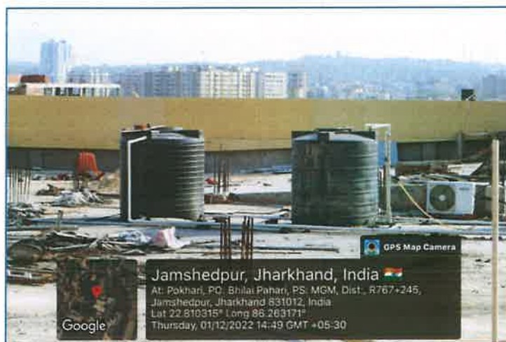
Water Tank: Chandra Shekhar Azad Block
