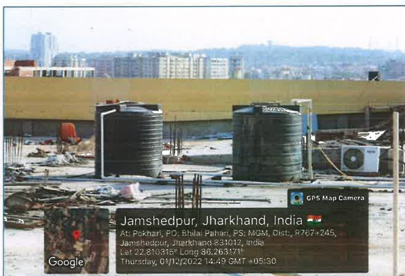
Water Tank: Chandra Shekhar Azad Block
